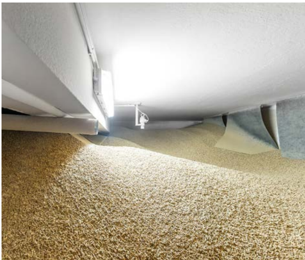
Im Gebäude liegender Pellets-vorratstank Pellet storage tank located in the building
